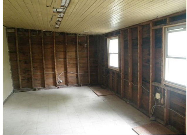
Figure 15: The upstairs office prior to renovations in 2010. Photo courtesy of Globe Productions
