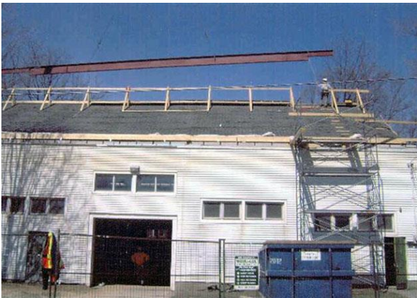
Figure 17: Roof reconstruction at the Old Armoury. Date between 2010-2015. Image Courtesy of Georgetown ON Magazine (georgetownon.ca)
