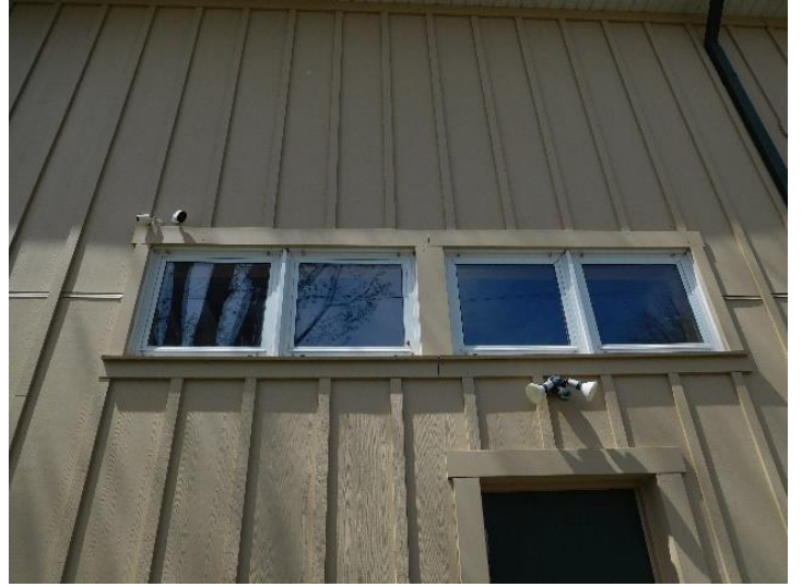
Figure 34: Detail of the double pane windows just above the side service entrance (Town of Halton Hills 2022)
