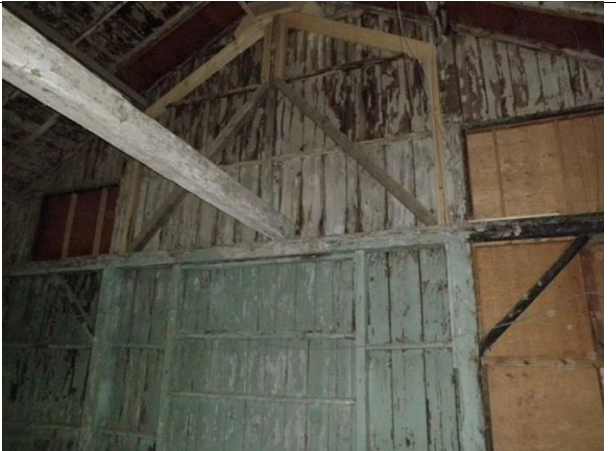
Figure 13: Interior of the Armoury prior to renovations. 2009. The original board-batten had been previously whitewashed and not maintained. Photo Courtesy of Globe Productions
