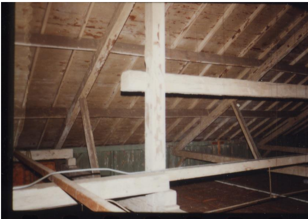
Figure 43: Photo of the roof trusses taken by the Department of National Defense. (EHS12567)
