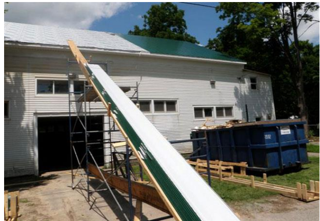
Figure 18: Old roof being replaced with green steel. Date between 2010-2015. Image courtesy of Georgetown ON Magazine (georgetownon.ca)
