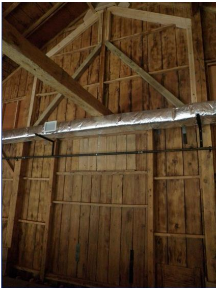
Figure 46: East interior wall of the main room of the Armoury. Image courtesy of Globe Productions
