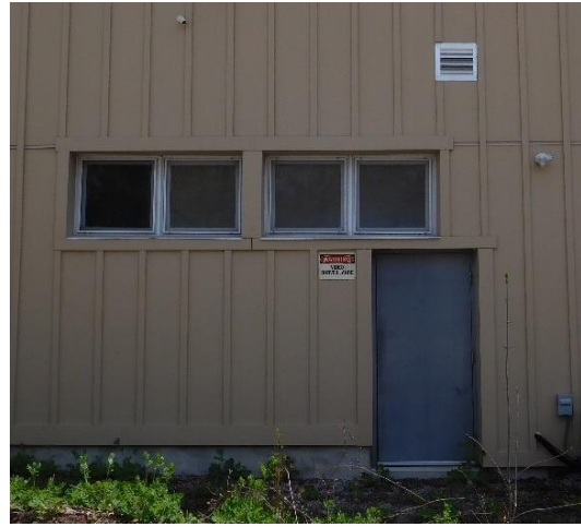
Figure 40: The door and windows on the rear elevation (Town of Halton Hills 2022)
