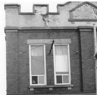
Figure 23: A 1996 photograph showcasing details of the second floor of the Starkman Block constructed in 1922. (EHS 23571)
