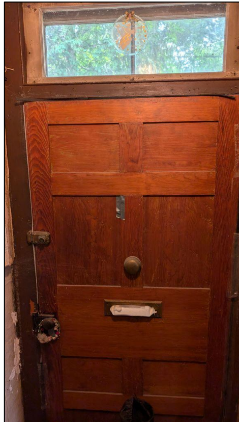
Figure 31: Wooden front door and transom found on the side (west) elevation of the existing dwelling (John Mark Rowe 2024)
