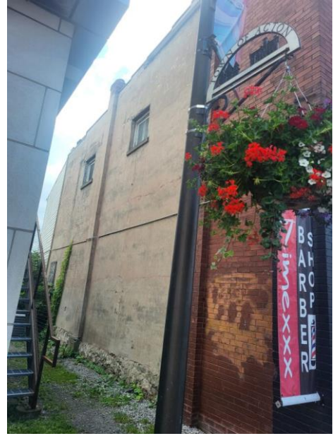
Figure 39: Looking along the northeast elevation of the existing building within the subject property from Mill Street East (Town of Halton Hills 2024)
