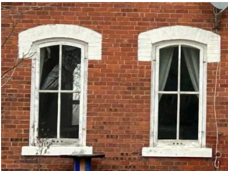
Figure 28: Segmentally arched window openings with painted brick voussoirs and stone sills at the first storey (Town of Halton Hills 2024)
