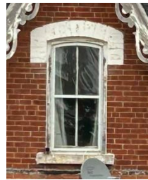
Figure 30: Second storey segmentally arched window opening with painted brick voussoirs and stone sills under central gable peak (Town of Halton Hills 2024)
