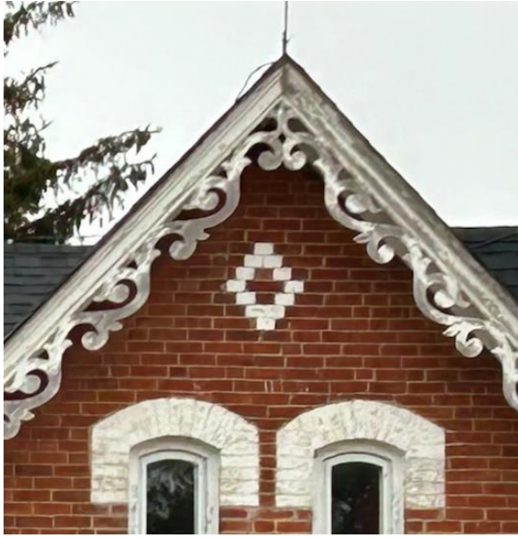
Figure 26: Decorative wooden bargeboard, finial, and white lozenge pattern directly above the bay on the front (southwest) elevation (Town of Halton Hills 2023)
